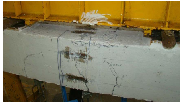
(b) final cracking at ultimate load
