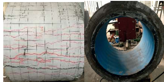
Fig. 16 – Crack distribution and RCP repaired with HDPE liner [91]
