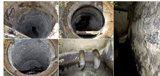
Fig. 3 – Photos of MIC in sewage facilities [17], Photos (A), (B), (D) are taken from the manhole of sewage pipes; Photos (C) and (E) are taken from wastewater catchment basins.
