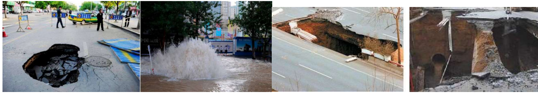
Fig. 2 – Pavement collapse and pipe burst caused by concrete pipes failure [7,8]
