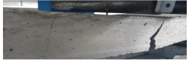
Fig. 16 – Control prism failure
