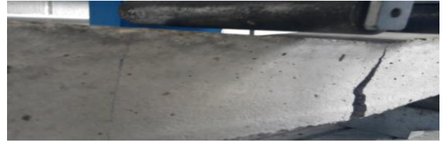
Fig. 16 – Control prism failure
