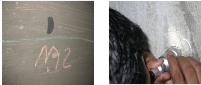
Fig. 1 – Crack measurement on upstream and downstream side of upper gallery-3
